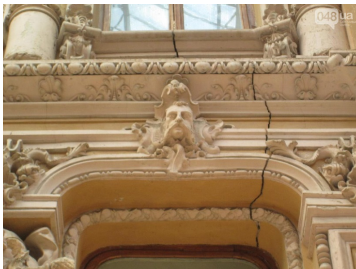
Pic 3. «Opened cracks on the facade of the "Passage"»
